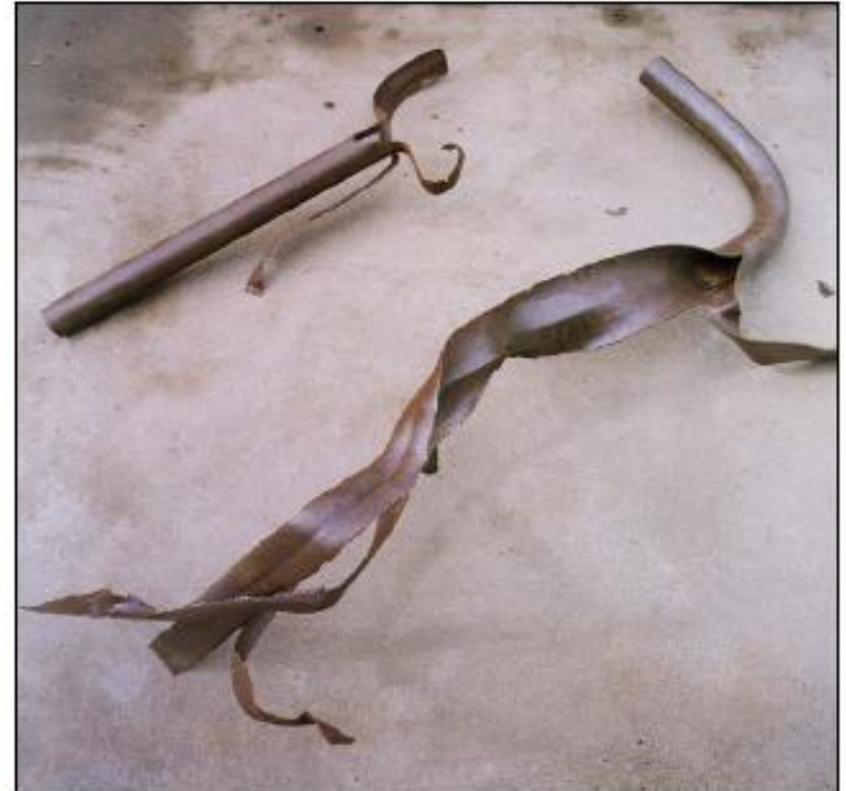
Organic peroxide contained in pipe
